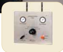
Nitrogen control panels
